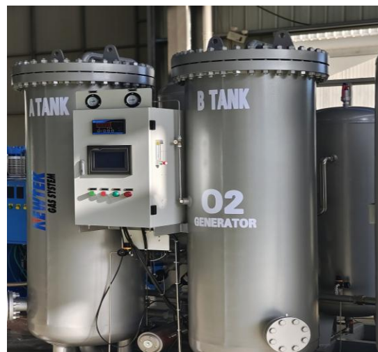
Twin Tower PSA System
